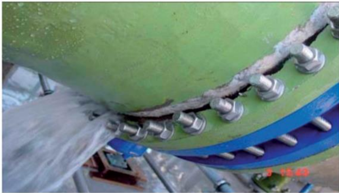
Figure 1: Corrosion effect (rusting) on metallic flange [12].
